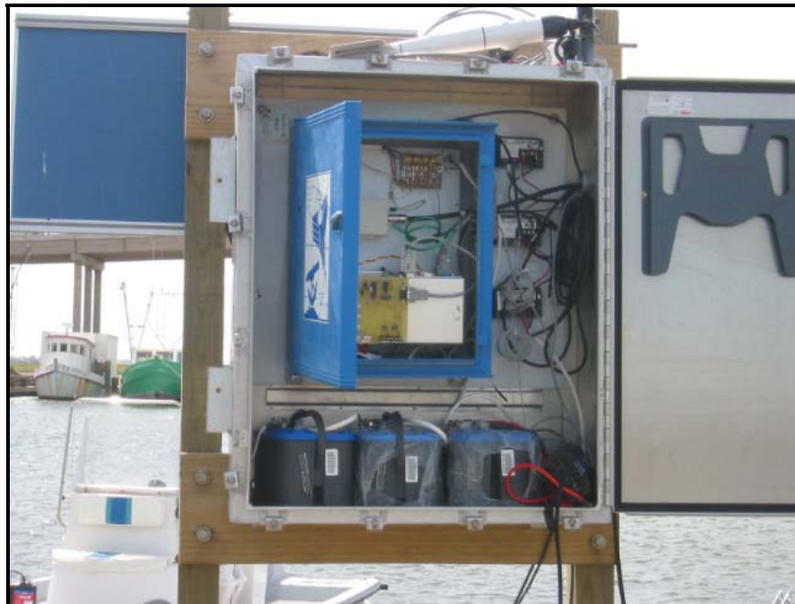
Figure 14. Photo of the components of the data controller/logger/telemetry box.
