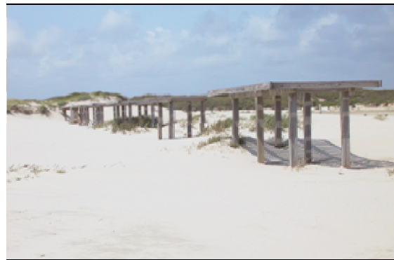
Figure 11. Wind-blown sand covering picnic facilities at Mustang Island State Park (September 2003).
